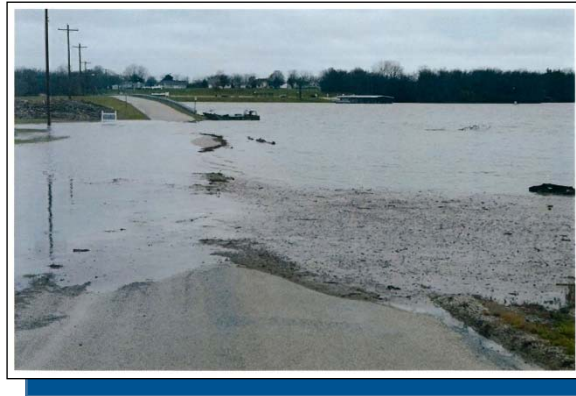
During the December 28, 2015 flash flood event, Glenn Shoals Lake overtopped Glenn Shoals Drive as the emergency spillway was utilized to handle the excess water.
