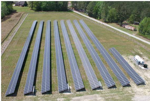
▲ Double Eagle Solar and Storage, North Carolina, 0.7MW with a 500kW/1000kWh Battery Energy Storage System (BESS)
